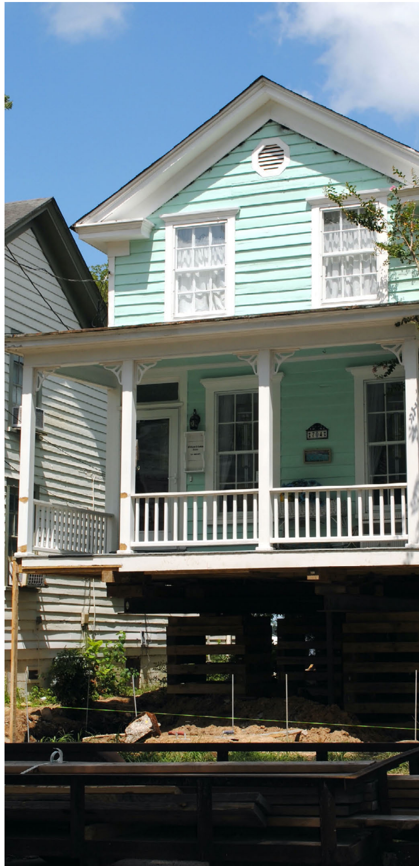
A new brick foundation with piered brick panels was constructed to elevate this New Bern house and its front porch approximately 5 ft. above grade. Courtesy of the State Historic Preservation Office, North Carolina Department of Natural and Cultural Resources.
