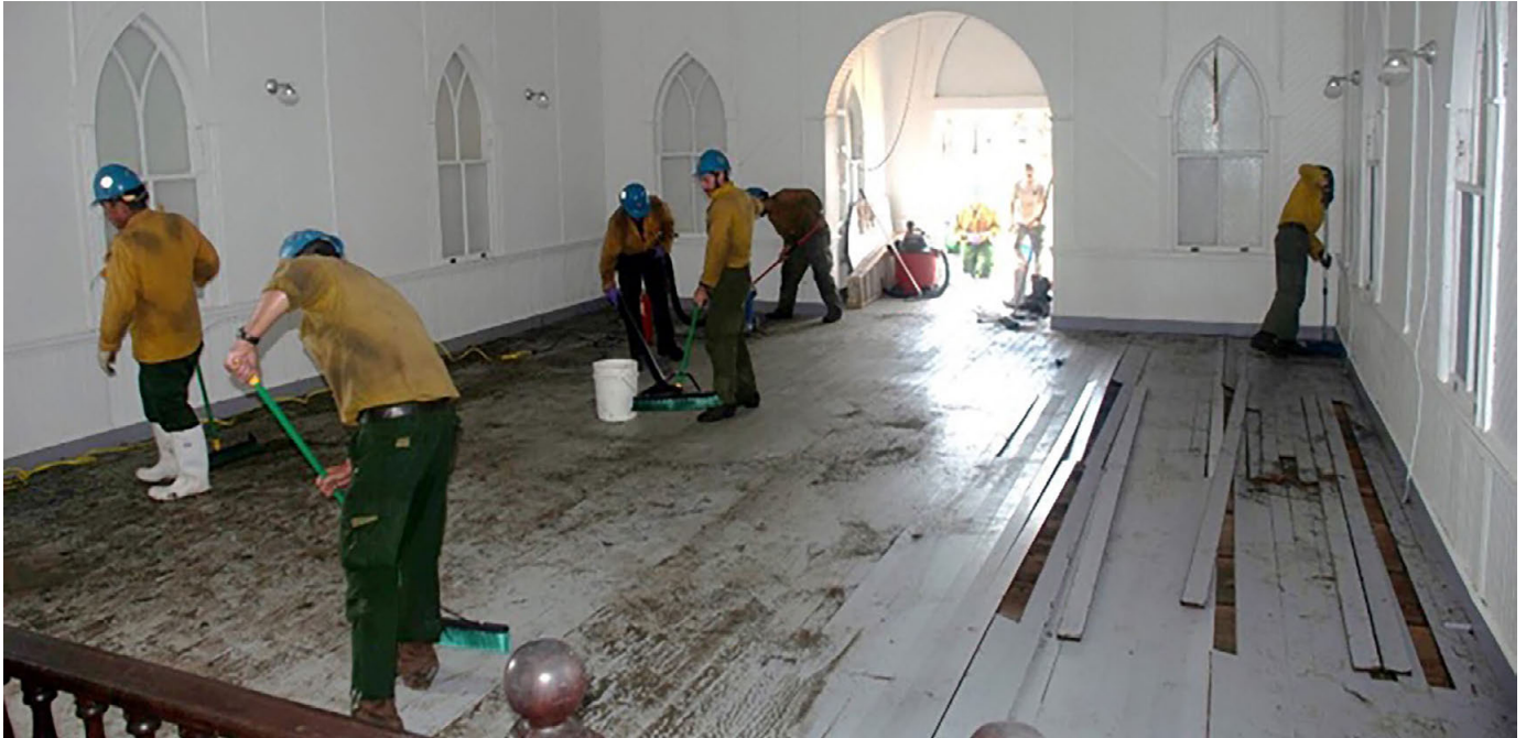
As flood waters receded post–Hurricane Dorian, pressure from the flood water trapped inside the Methodist Church on Portsmouth Island buckled sections of the flooring as the water sought to escape. After the interior was cleaned and dried out, the floors were repaired and trap doors were installed in the floor to provide a path for future flood waters to drain out. Courtesy of Jeff West, Cape Lookout National Seashore.
