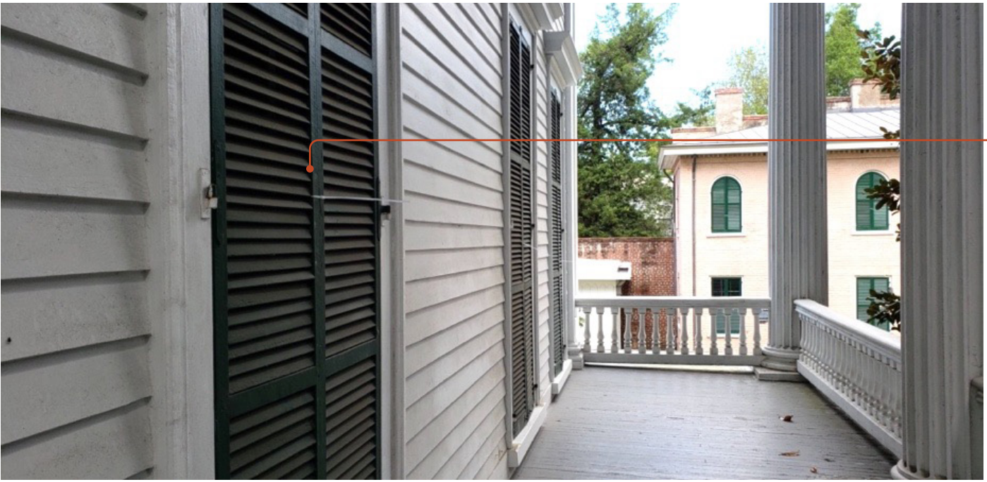
The operable wooden shutters on the Bellamy Mansion (in foreground) and its slave quarters (in background) in Wilmington are routinely closed and secured in anticipation of hurricanes to protect the windows and interior from storm damage. Courtesy of Bellamy Mansion Museum.
