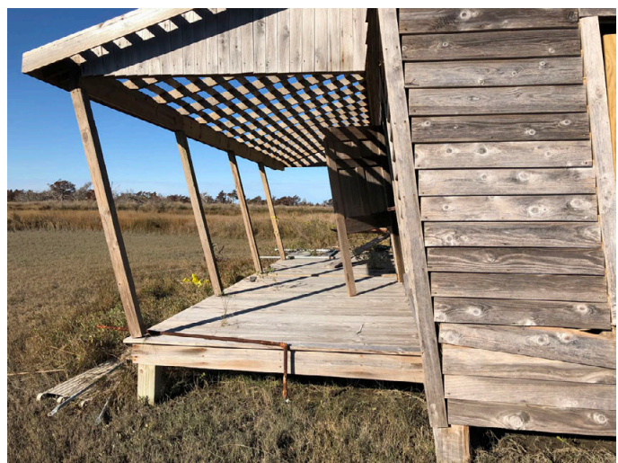
Strong wind from Hurricane Dorian in September 2019 caused shearing along the foundation of the George Dixon House in Portsmouth Village. Courtesy of Jeff West, Superintendent of Cape Lookout National Seashore.
