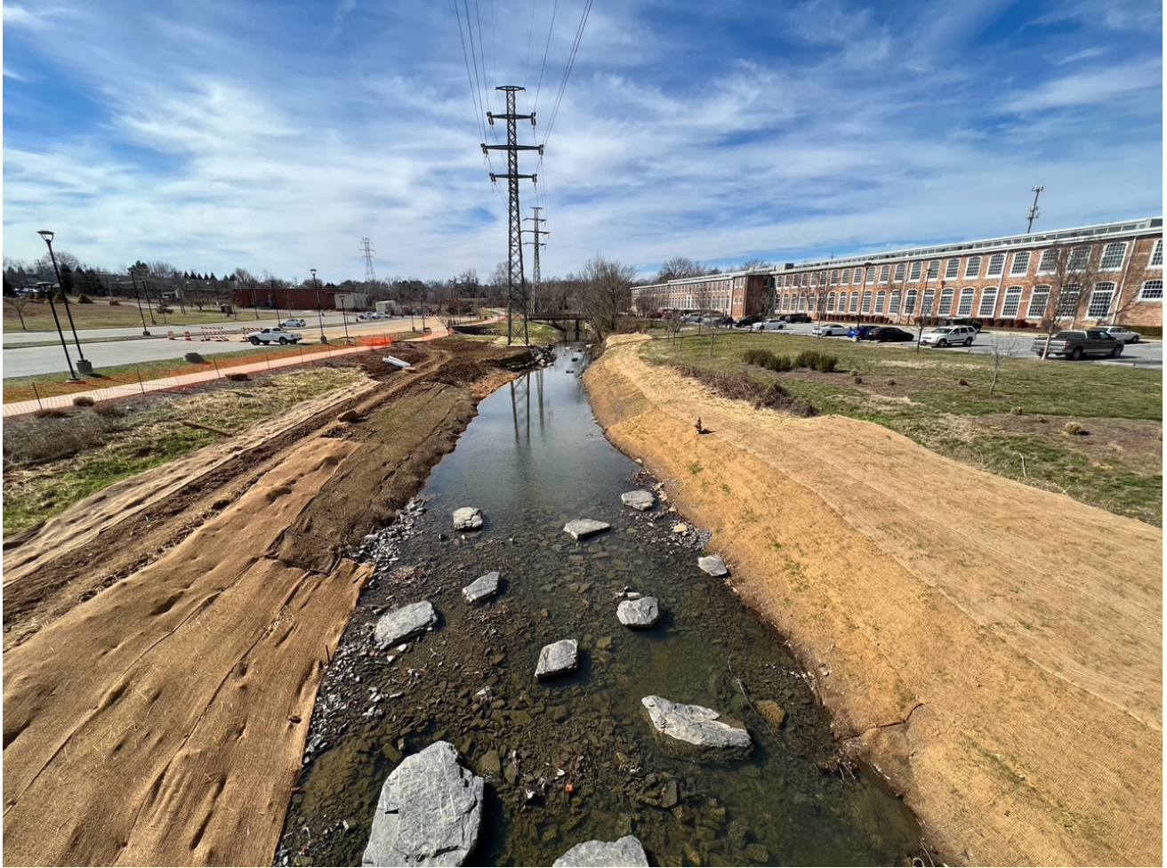
Restoration of Buffalo Creek on the Revolution Mill campus in Greensboro involved removing debris from the creek, terracing the banks, and installing large rocks to slow the stream flow at key points—all of which will help mitigate future flooding. Courtesy of Eddie Belk, Belk Architecture.
