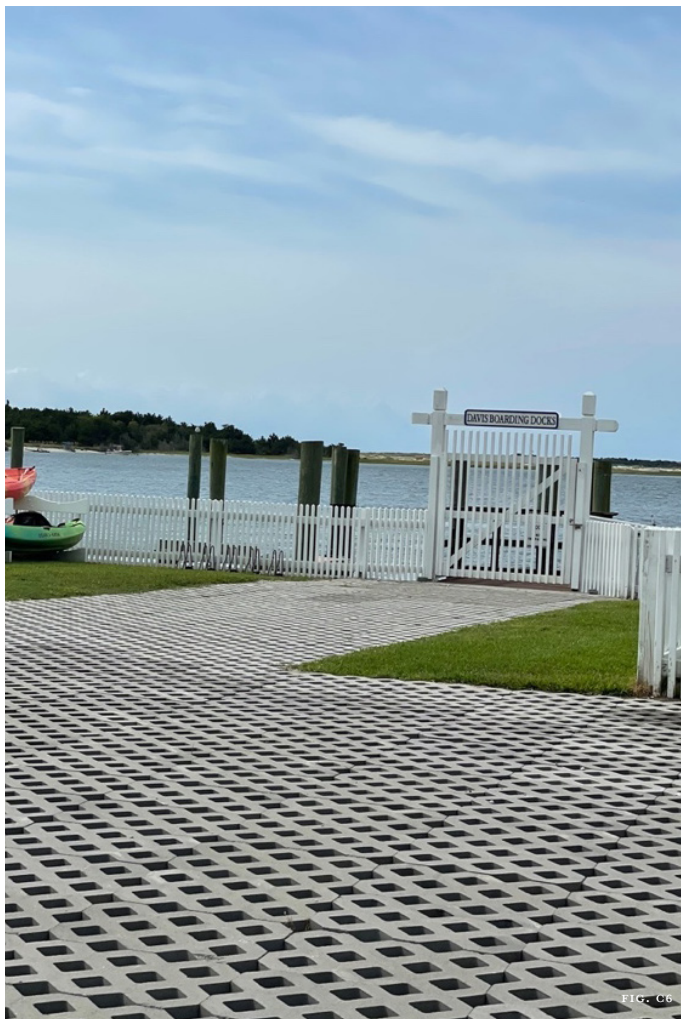
Figure C6: Concrete paver modules have been installed to create a permeable parking surface for accessing this dock in Beaufort. The openings in the modules can be filled with gravel or plantings.
