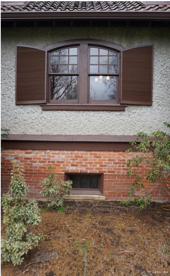
Figure H1: Original, recessed windows in the foundation of the Biltmore Gardener's Cottage were retained when the foundation was raised, and they continue to provide daylight, as well as ventilation when opened, to the basement space.
