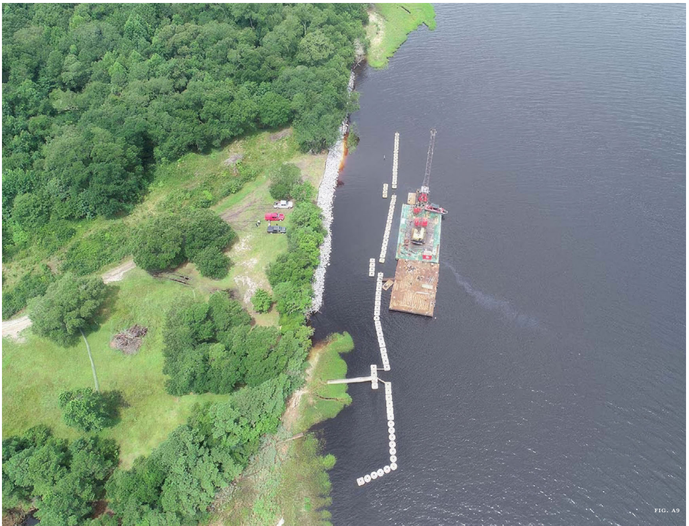
Figure A9: An aerial view of the attenuators installed in the Cape Fear River at Brunswick Town /Fort Anderson State Historic Site to stop naturally occurring erosion and absorb wave energy from international shipping while allowing for the eroded shoreline to be rebuilt with sedimentation.
