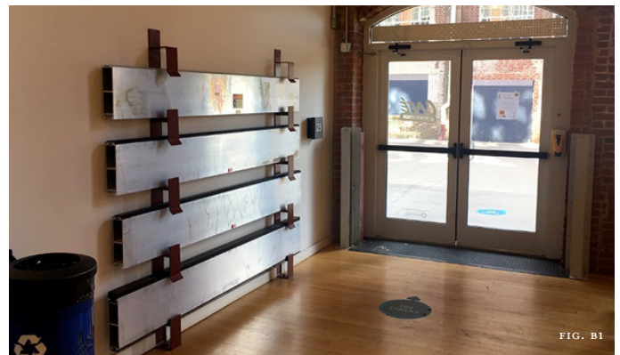
Figure B1: At Revolution Mill in Greensboro, temporary floodgate slats are stored on brackets close to the entry doors for quick access in anticipation of flooding.
