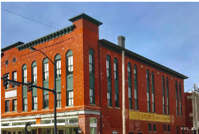
Figures K1 and K2: In Elizabeth City, Hurricane Isabel seriously damaged the built-up roof of this historic commercial building, resulting in substantial interior damage as well (above). It has since been fully rehabilitated (below).
