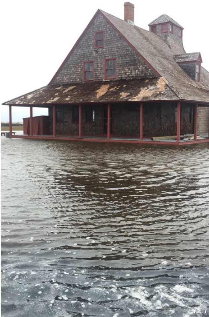
Figure 1: Sequentially, Hurricanes Florence and Dorian severely damaged properties in Portsmouth Village on Cape Lookout National Seashore. The National Park Service has since completed repairs to the Lifesaving Station and multiple other historic structures.
