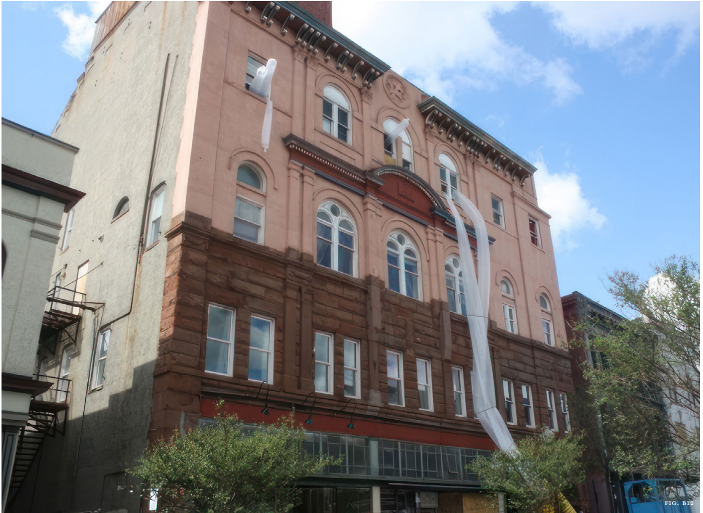
Clockwise from top left— Figure B8: Plywood panels provide temporary protection for window openings and exterior wall areas of this New Bern house damaged by Hurricane Florence. Figure B9: Wooden elements retained in place after being inundated with over 30-inches of floodwaters at Williams Hall on the Carolina Industrial School campus were slowly dried out and treated with a borate preservative to deter future mold growth and insect damage. Figure B10: The damaged gable roof of the Tileston School in Wilmington was temporarily protected by the installation of a synthetic rubber roofing membrane. Figure B11: Corrugated drainpipe extensions were used to temporarily carry rainwater further away from the foundation of this Edgecombe County house. Figure B12: Low heat and a dehumidification system were utilized to dry out the Masonic Building in Wilmington after flooding.
