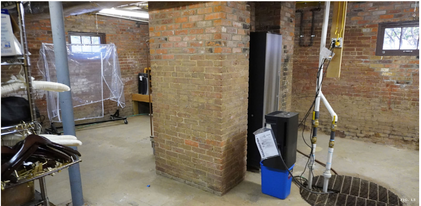
Figure L1: A ductless mini-split system mounted on a sturdy platform above the established flood risk level of this property on the sound in Atlantic increases its resilience to flooding. Figure L2: Mechanical ductwork, plumbing lines, and electrical lines were all moved higher when the Biltmore Market Gardener’s Cottage was elevated. Water heaters and stored items were also raised at least a foot above the basement floor to prevent potential water damage. Figure L3: Sealed foundation vents, a sump pump, a dehumidifier, and a central drain reservoir all work to eliminate moisture in this basement.
