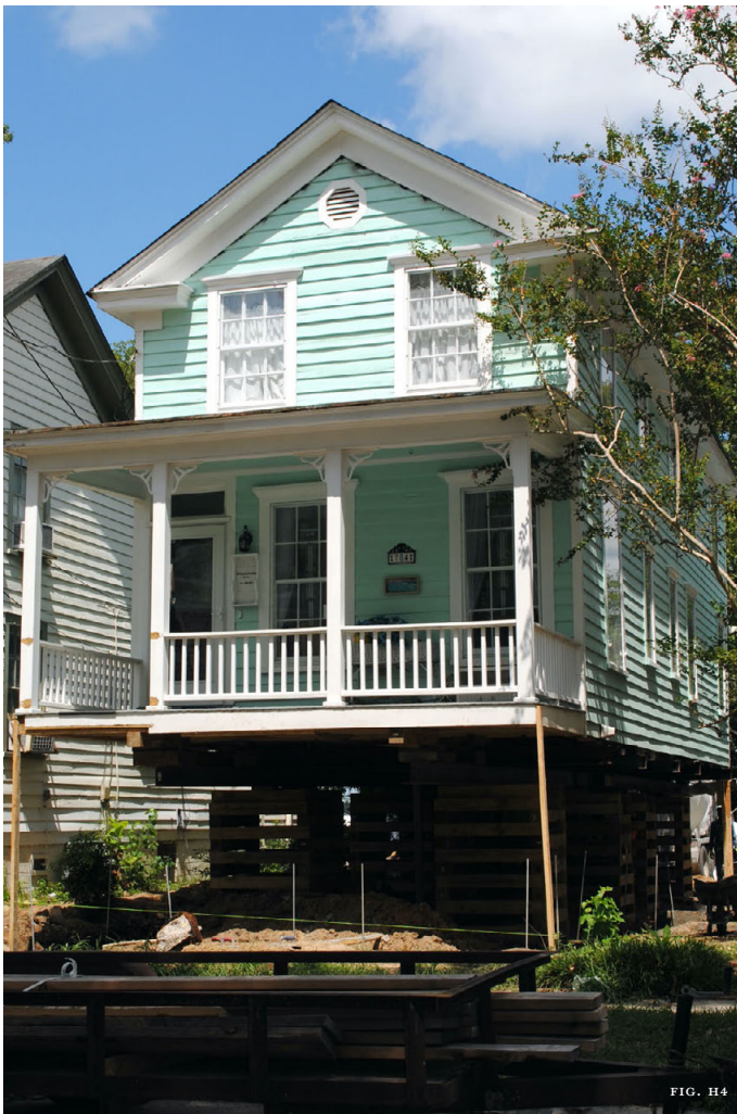
Figure H4: A new brick foundation with pierced brick panels was constructed to elevate this New Bern house and its front porch approximately five feet above grade.
