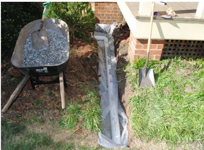
Figure A2: A French drain installed at the Joel Lane House in Raleigh funnels stormwater away from the perimeter of the building foundation and front porch.
