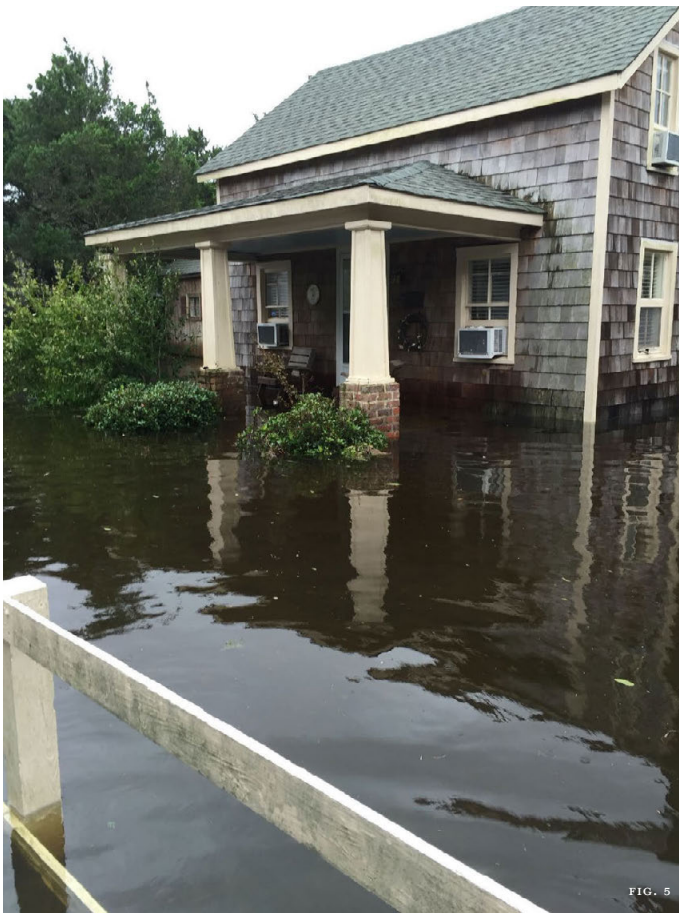
Figure 5: Vernacular cottages along the N.C. coast like this Ocracoke house seen in 2016 after Hurricane Matthew are flooding with greater frequency during severe weather events. This house was elevated in 2017 and successfully weathered Hurricane Ian.
