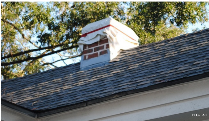
Figure A1: Because this chimney is not capped, it was temporarily covered with waterproof material to prevent water intrusion.
